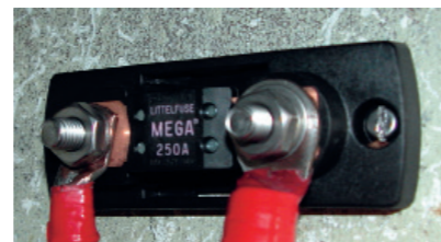
A typical high-current battery fuse at the primary source of power
