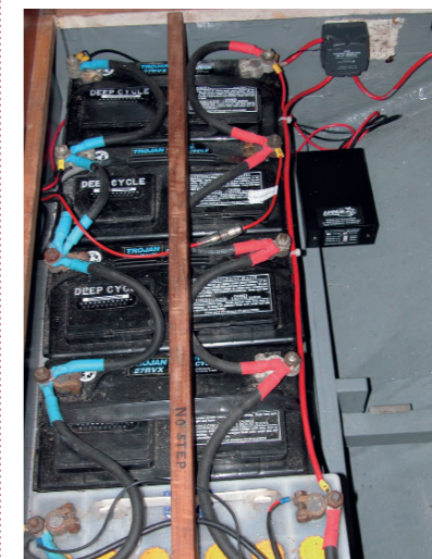
If your batteries are in a bank, they all need changed at the same time
