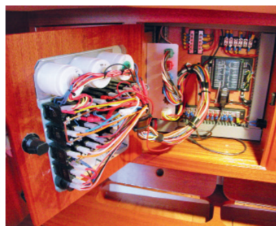
Marine-grade wires, cables and electrical components should be used on board
